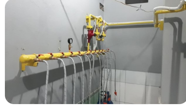
Instalasi Pipa Gas
